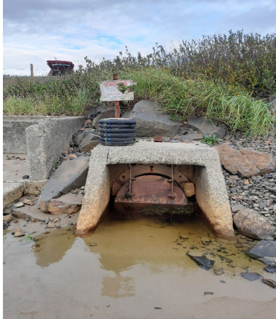
Figure 9: Photo of outfall at Site 36621 that connects Chisana Creek to Tolovana State Beach.
