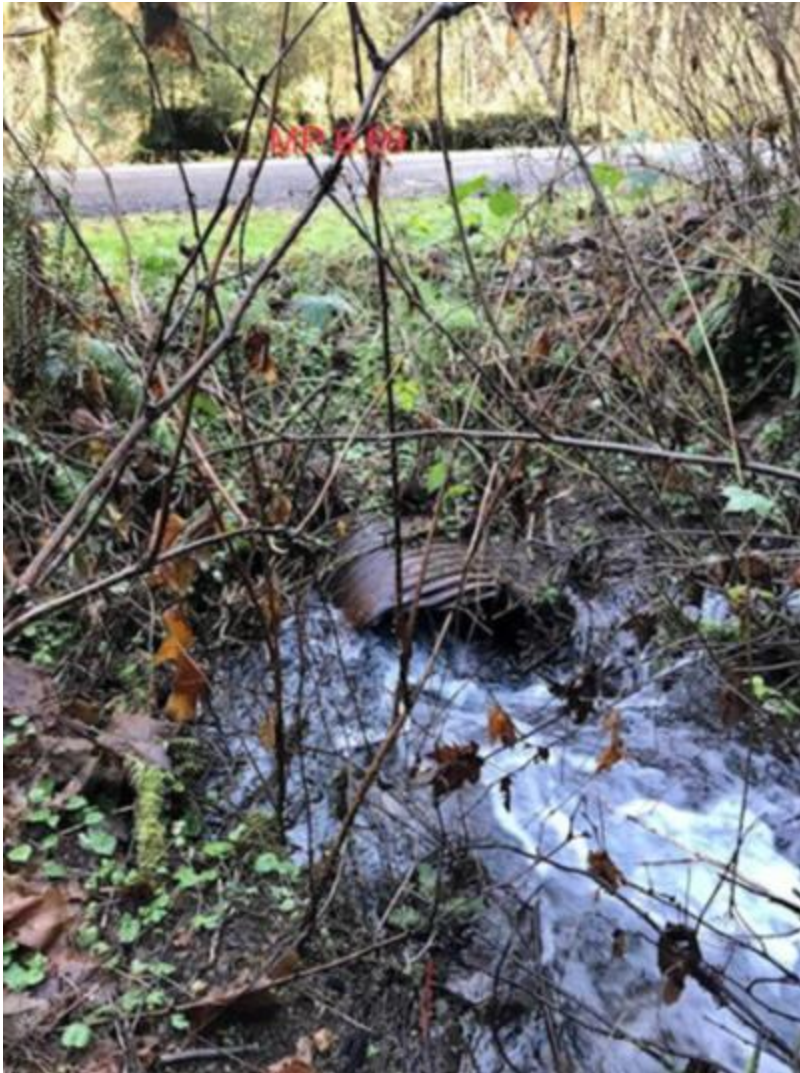
Before: Undersized culvert at mile post 6.69
