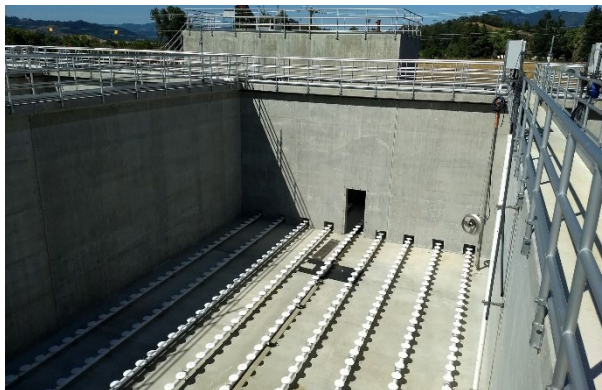
Wastewater aeration basin
