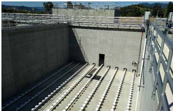
Wastewater aeration basin
