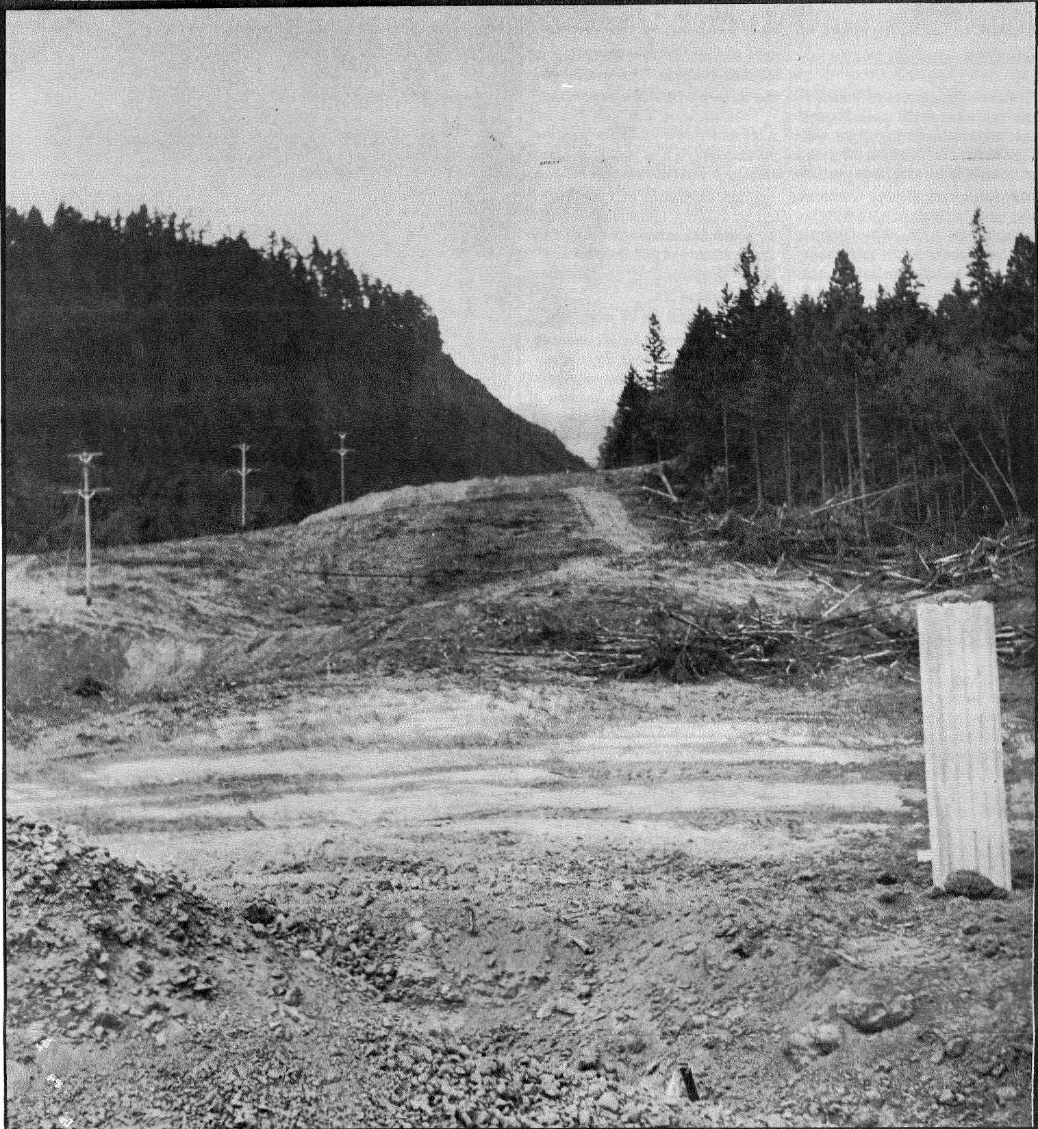
CLEARING FOR TRAM LINE TAKEN FROM ORE STORAGE. MINE TOP CENTER OF PICTURE.
