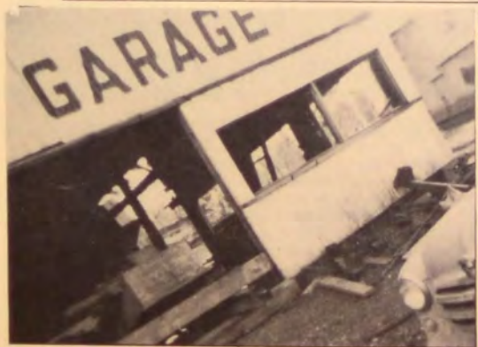
THIS GARAGE BUILDING IS BEING CONVERTED INTO A CHROME CONCENTRATING MILL BY HELMKE, THOMAS AND JANSSEN, ROLL CRUSHER NOTED IN DOORWAY. OPERATION UNDER MANAGEMENT OF JIM McDONALD OF MAGALIA. MINE IS LOCATED ABOUT 4 MILES WEST OF MILL. UPON COMPLETION MILL WILL HAVE AN APPROXIMATE 50 TON DAILY CAPACITY OF HIGH GRADE ORE.
