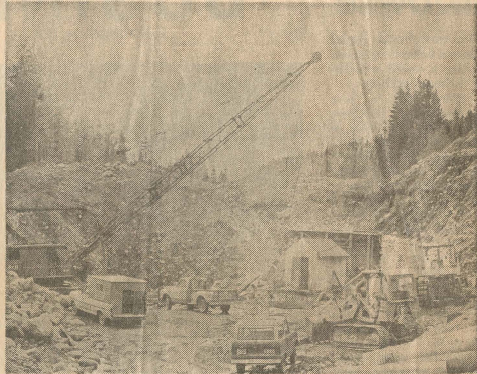
OPEN PIT — Cornucopia Minerals mining operation near Halfway looks like highway project Crane (left) digs into
