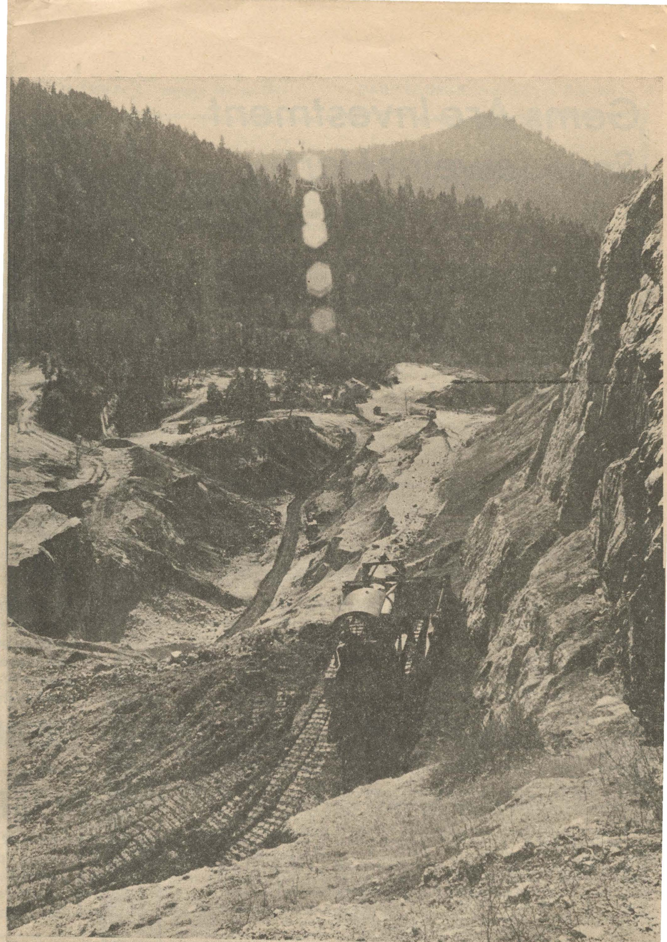
ACCESS to the blasting site for new excavation at the Bristol Silica mine on Miller Creek is leveled by Bud Ross.
