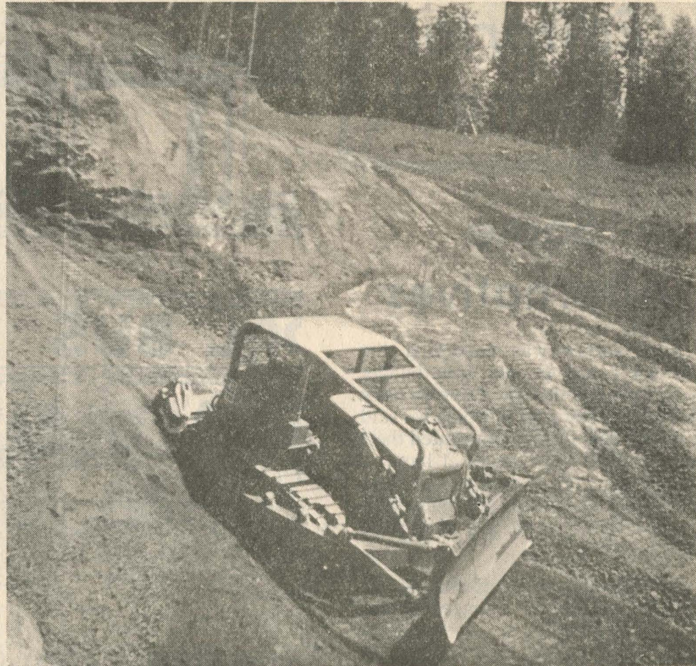
CATERPILLAR clears route in pit in zones in background in white. picture taken from uphill side. Note the ore
