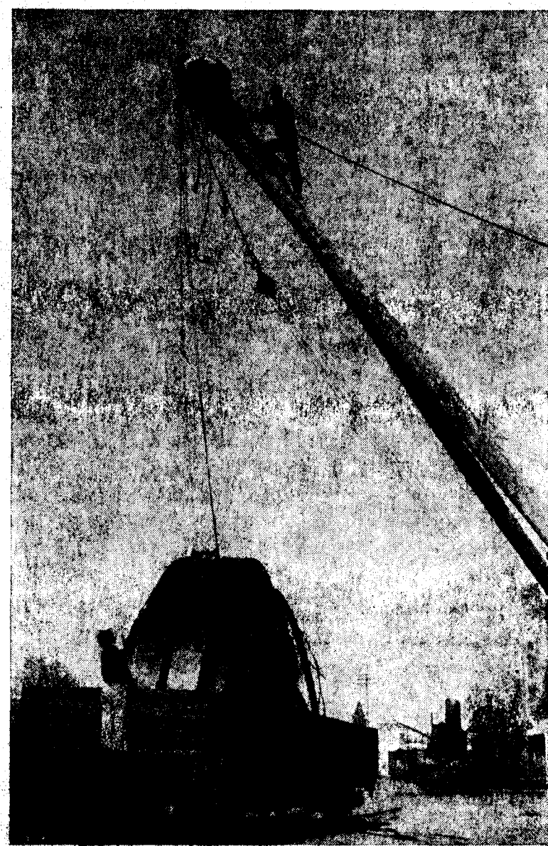
Dragline dredge equipment of such size that seven or eight freight cars are required to bring it here from the Merriam Manufacturing company in Ohio was being shifted to a truck at the local yards Friday morning to be taken to Althouse creek, near Holland, for operations by the Atlas gold dredgers. Pictured here are two pieces for the pontoon, together weighing 28 tons. Yet to arrive are the Diesel-electric engine, 100-foot boom, five-yard bucket, cab, and other equipment which will bring the total weight to about 170 tons. The new machinery will replace a link belt dragline that the company has used on Althouse creek since setting up operations there several months ago. (Courier Photo and Engraving.)
