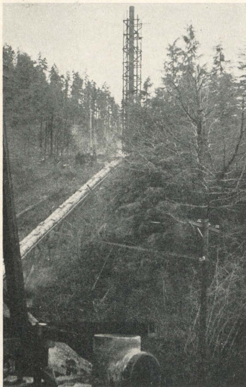
Stack flue and stack at the Black Butte quicksilver plant. The stack flue consists of twin lines of 15-in. tile pipe, leading up the slope to the stack. An air injector at the base of the stack aids in inducing draft. Oil is used for fuel, with the rather high consumption of oil due to high moisture content of the ore and the fairly coarse kiln feed.
