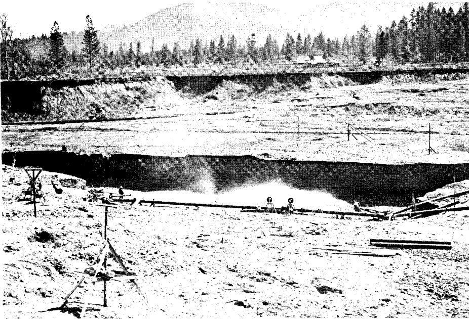
Figure 7. Giants similar to those described at checkpoint 28. These giants were operated in Josephine County, but similar ones were used in placer operations in the Bohemia district.
