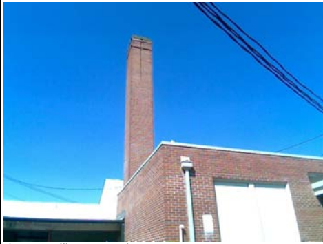
S Falling Hazard
