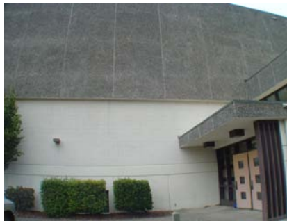
E Falling Hazard
