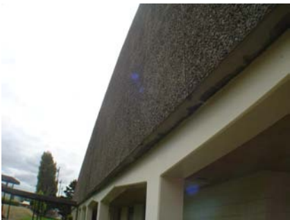
E Falling Hazard
