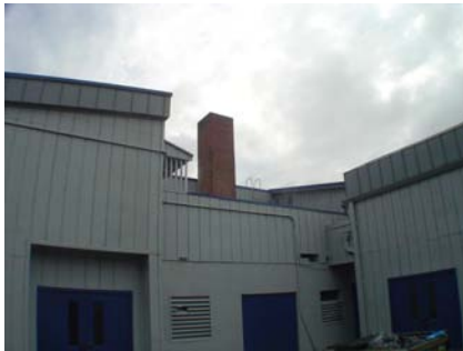
N Falling Hazard
