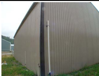
NW General Site
