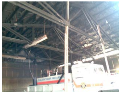
S Poor Condition fire damage
