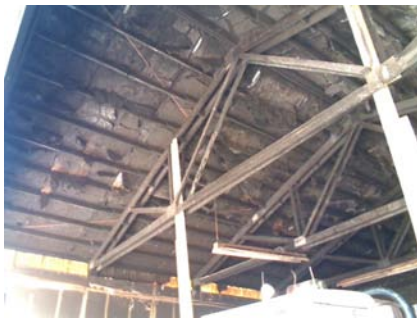
E Poor Condition fire damage
