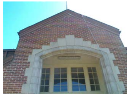
W Falling Hazard cladding
