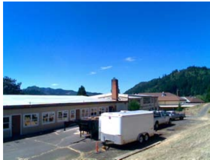
NE Falling Hazard chimney upgraded but not very well
