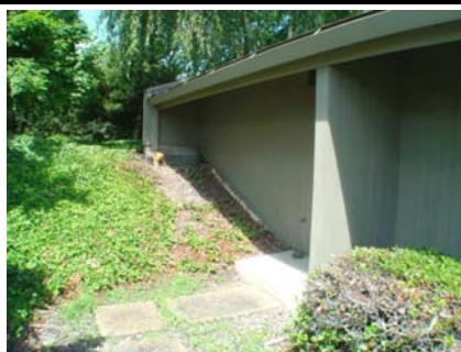
S Other About 10' of the building buried all along the west side.
