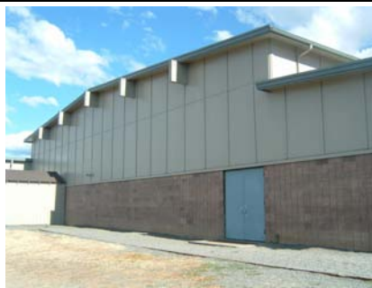
N General Site Shows RM1 for the lower part and W2 for the upper part. Also shows a vertical irregularity.
