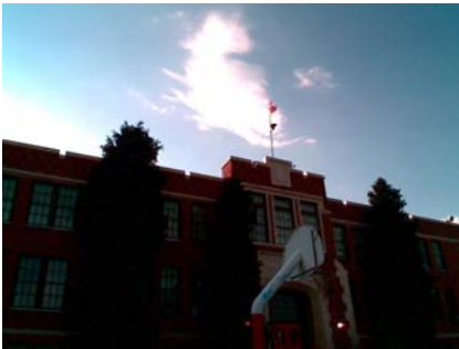
SE Falling Hazard partial upgrade?
