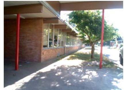
S Plan Irregularity Secondary shows approx 100ft of windows with walls on the other side indicating a possible torsion problem.
