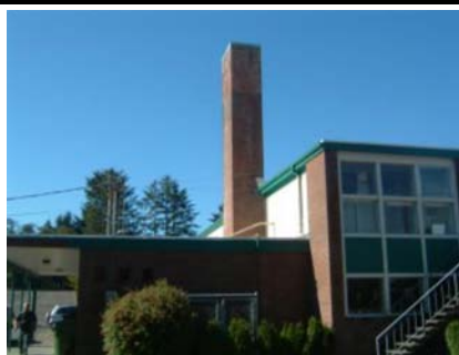
N Falling Hazard reinforced?
