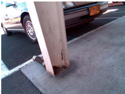
SW Building Quality building is bolted directly to slab
