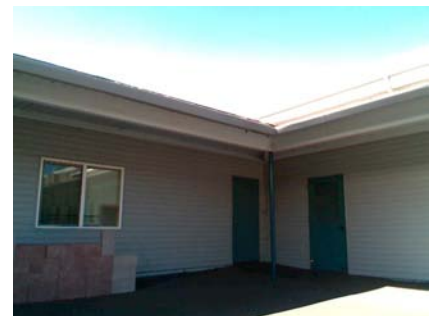
S Falling Hazard
