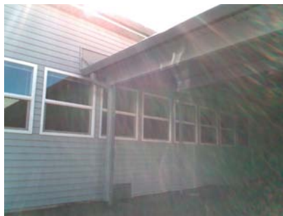
E Falling Hazard
