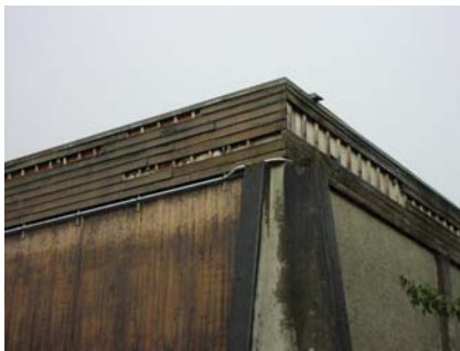
SW Poor Condition
