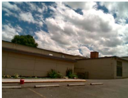
NW Falling Hazard
