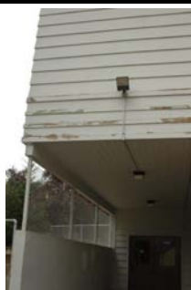
E Vertical Irregularity Tertiary some concern over these short columns - do they support gravity loads above?
