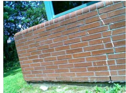
SW Poor Condition
