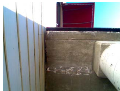
W Pounding Potential Looking up where walkway meets building.
