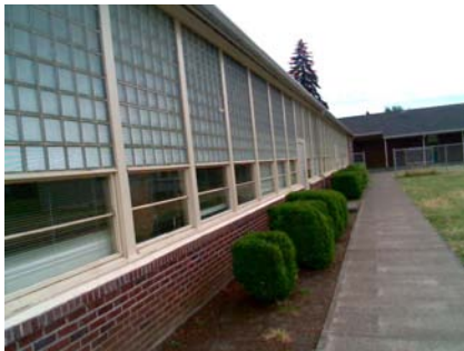
NE Falling Hazard brick and glass block
