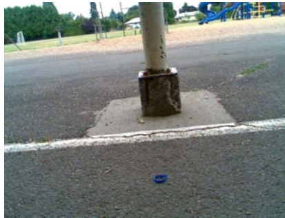
W Poor Condition base of column supporting covered play area. Full length of bolt exposed along the edge of the concrete.
