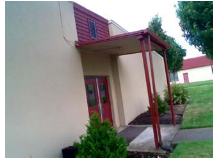
NW Falling Hazard
