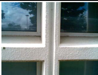
SE Primary Structural Type caulked gap
