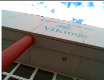
SE Falling Hazard Heavy concrete cladding
