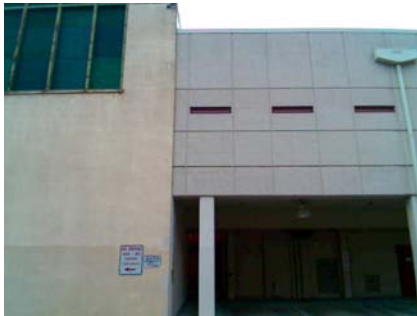
N Pounding Potential New const on right
