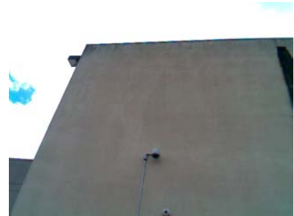
N Primary Structural Type small cracks show RM1
