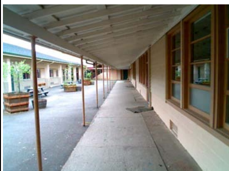
N Falling Hazard
