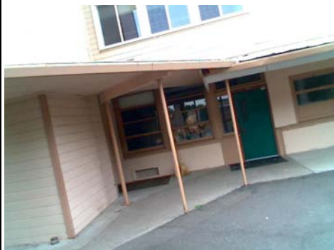
E Falling Hazard
