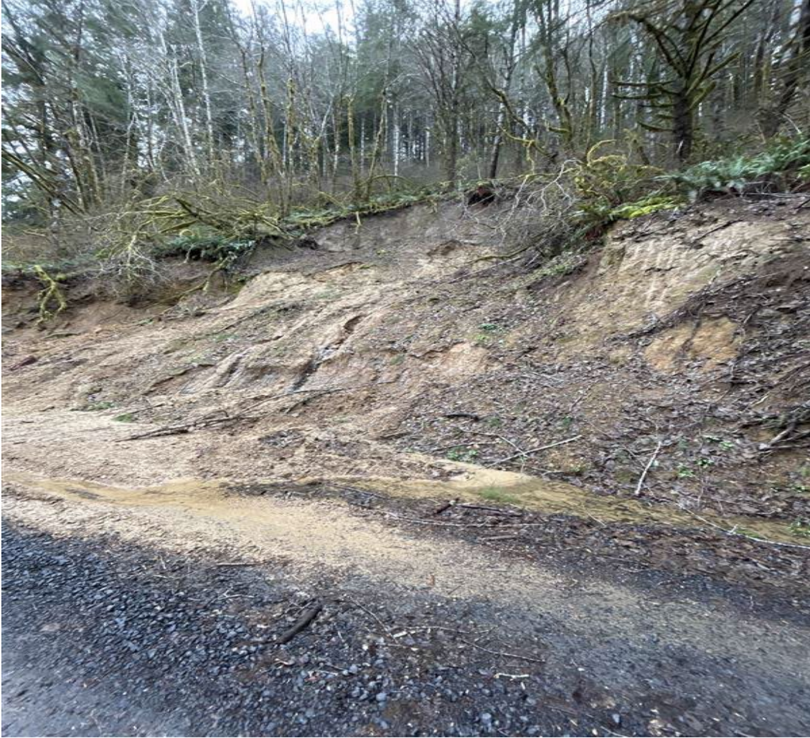
Figure 2.4.1. Slump delivering material onto 9000 road near confluence of Elk Creek and West Fork Millicoma River.
