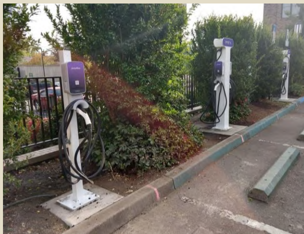
In 2020, the City of Ashland installed free public EV chargers using Oregon Clean Fuels Program credits.
