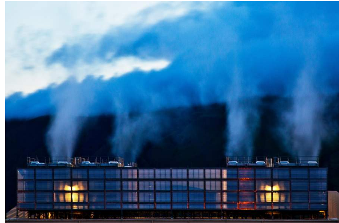
Steam rises above the cooling towers in The Dalles data center in Oregon. These plumes of water vapor create a mist at dusk. Google photo
