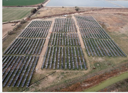
The City of Ontario’s Verde Light Oregon Community Solar project was the first completed Community Renewable Energy Grant-supported project.
