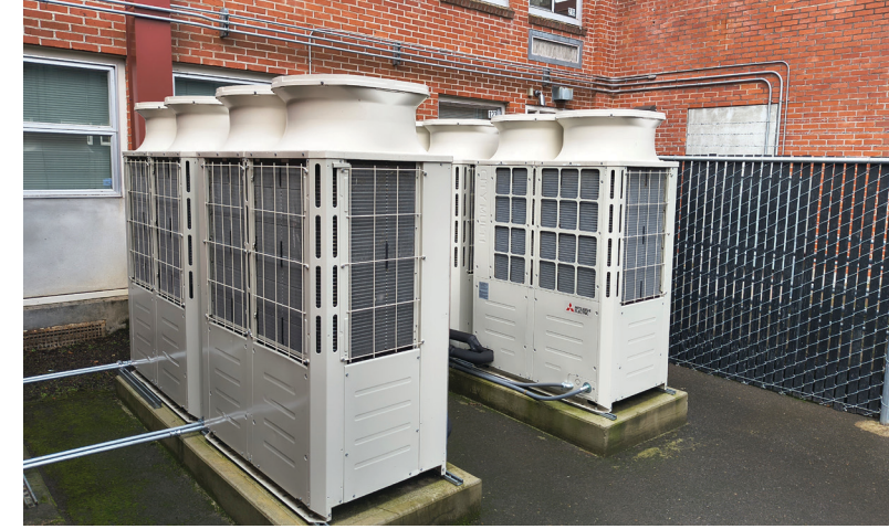
Heat Pumps at Estacada Middle School
