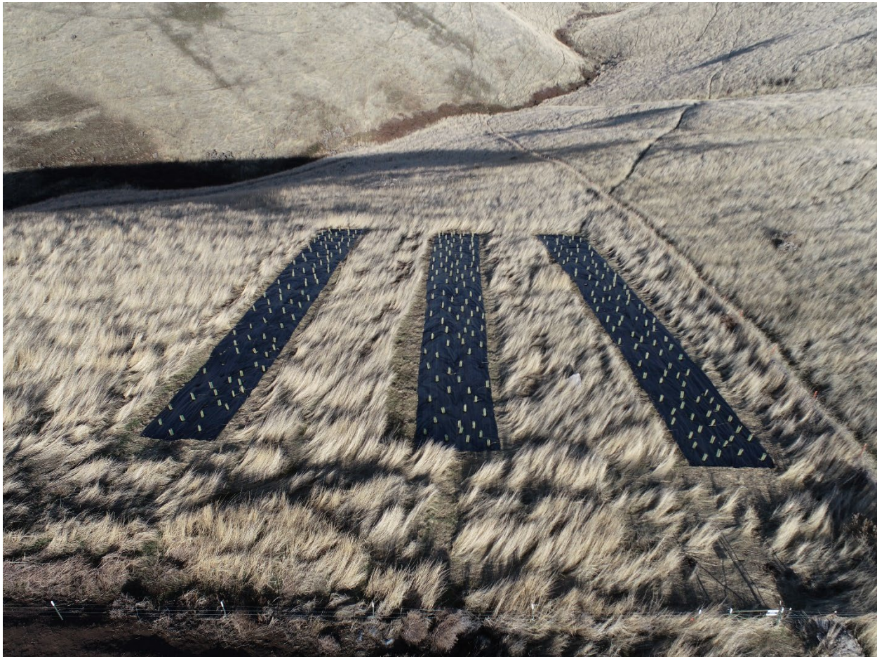
Figure 7. Aerial photograph of planted landscape fabric strips on hillslope adjacent to the spring site.
