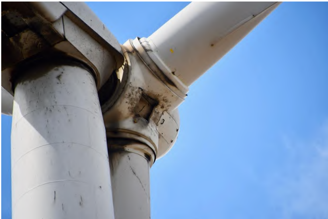
A Vestas V82 turbine, missing a hatch door, at PGE's Biglow Canyon wind farm this summer. Farmers say the hatches fall into their fields from a height of 265 feet. (Courtesy Kathryn McCullough)
