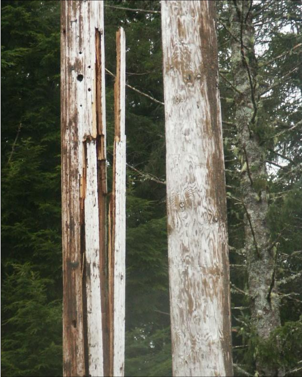
Figure 2.6. Cracked pole – an example of the type of conditions tree crews should report.
