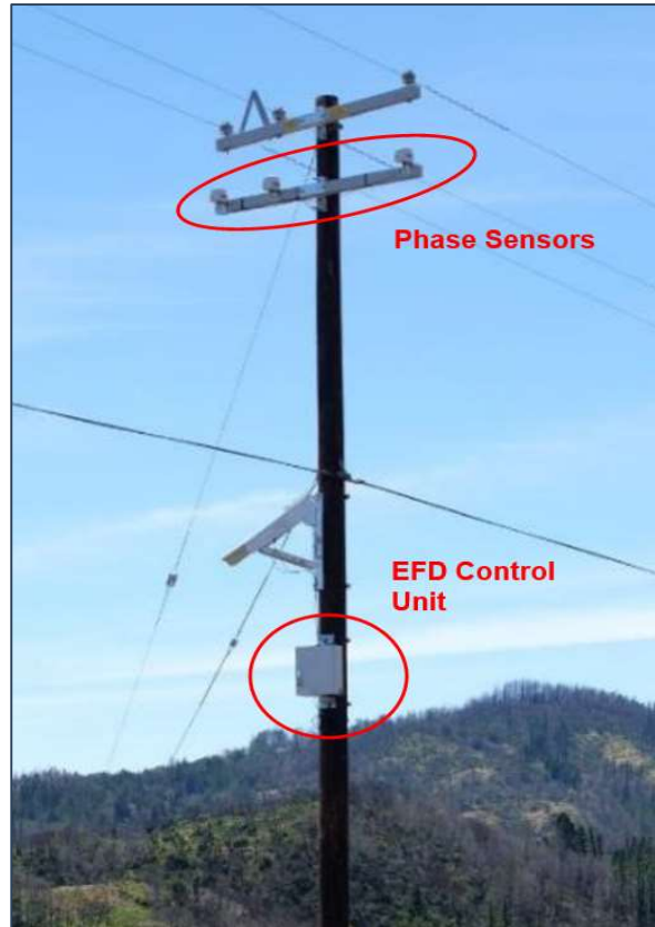
Figure 22: Example of An Installed EFD System
