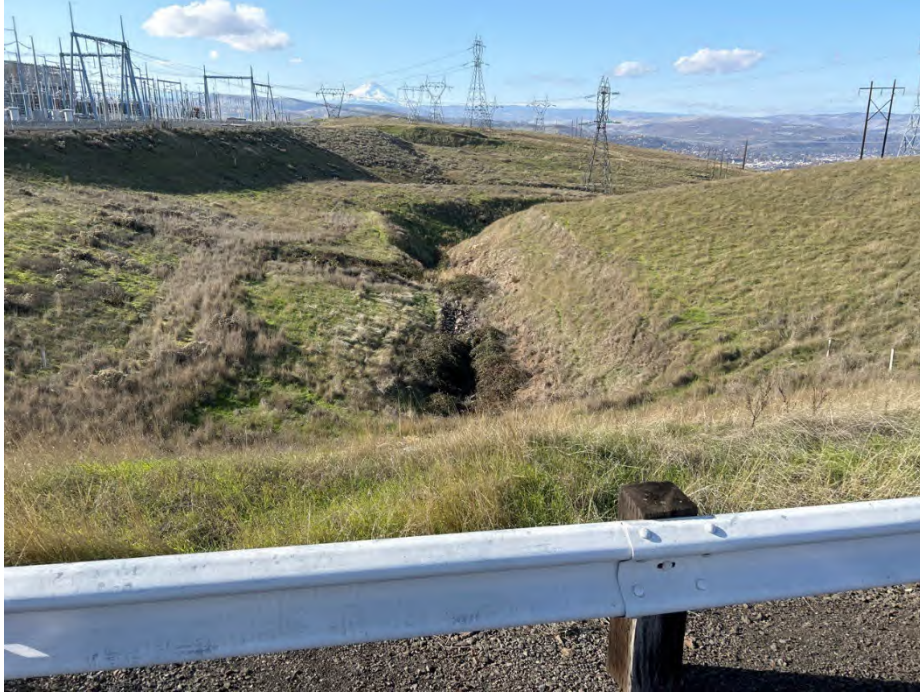
Photo 3a Looking downstream at an ephemeral drainage (Drainage 1) beneath Columbia View Drive, culvert occurs roughly 75 feet below road grade. Date: 11/08/23 Direction: Southwest
