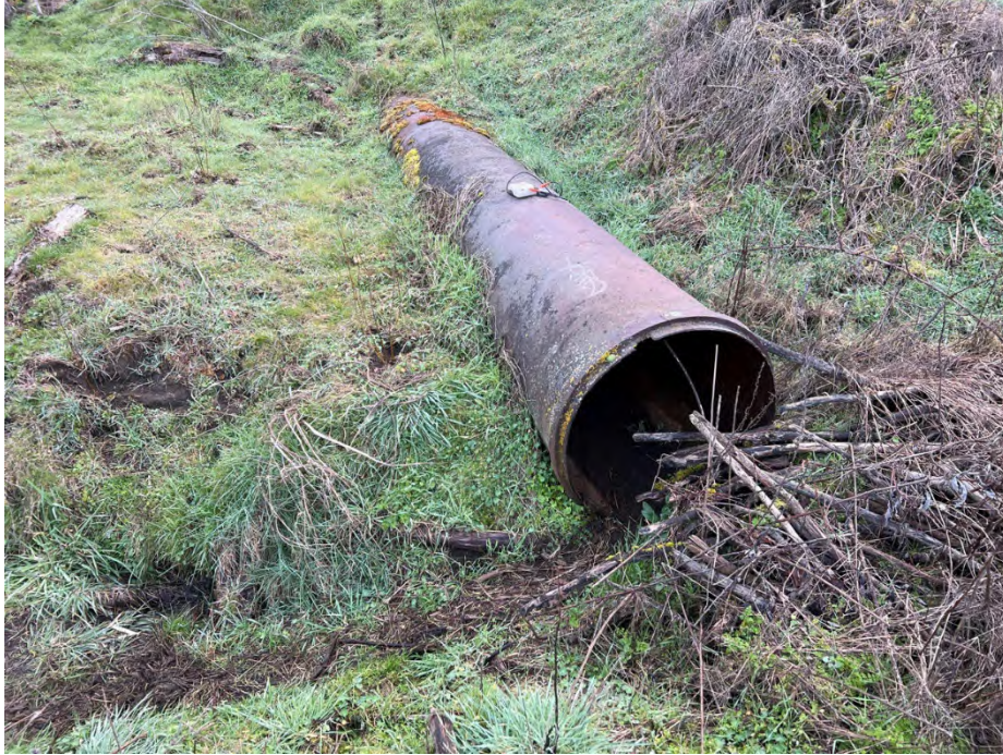
Photo 32 Roughly 24-inch culvert inlet to Wetland 3; a large stormwater feature. Signs of recent flow observed. Date: 03/13/24 Direction: East
