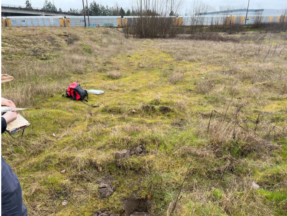
Photo 26 Sample Plot Area B-P1 (W) taken within suspect depressional area in human-made stormwater feature with no outlet. Geomembrane liner encountered 12 inches below ground surface. Date: 03/11/24 Direction: Southwest
