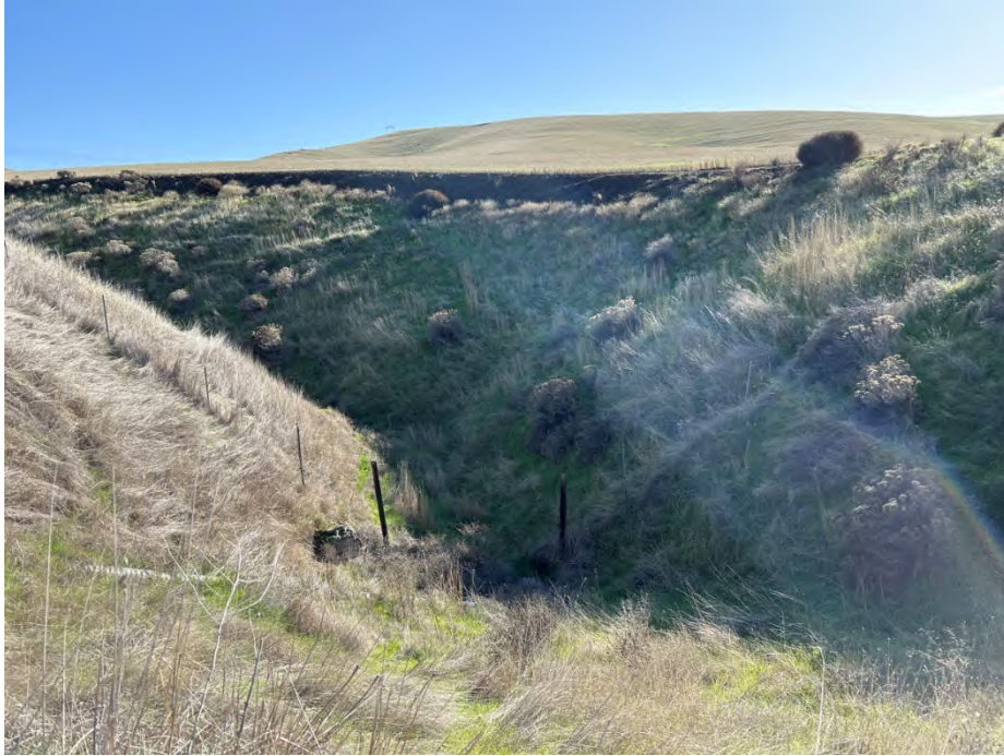
Photo 4a Looking upstream at an ephemeral drainage (Drainage 2) to Threemile Creek beneath Columbia View Drive; culvert present roughly 30-40 feet below road grade. Date: 11/08/23 Direction: East
