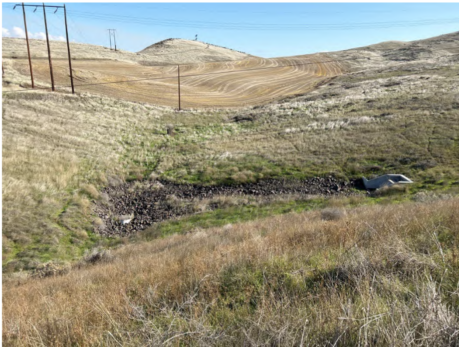
Photo 3b Looking upstream at an ephemeral drainage (Drainage 1) beneath Columbia View Drive, culvert occurs roughly 75 feet below road grade. Date: 11/08/23 Direction: Northeast
