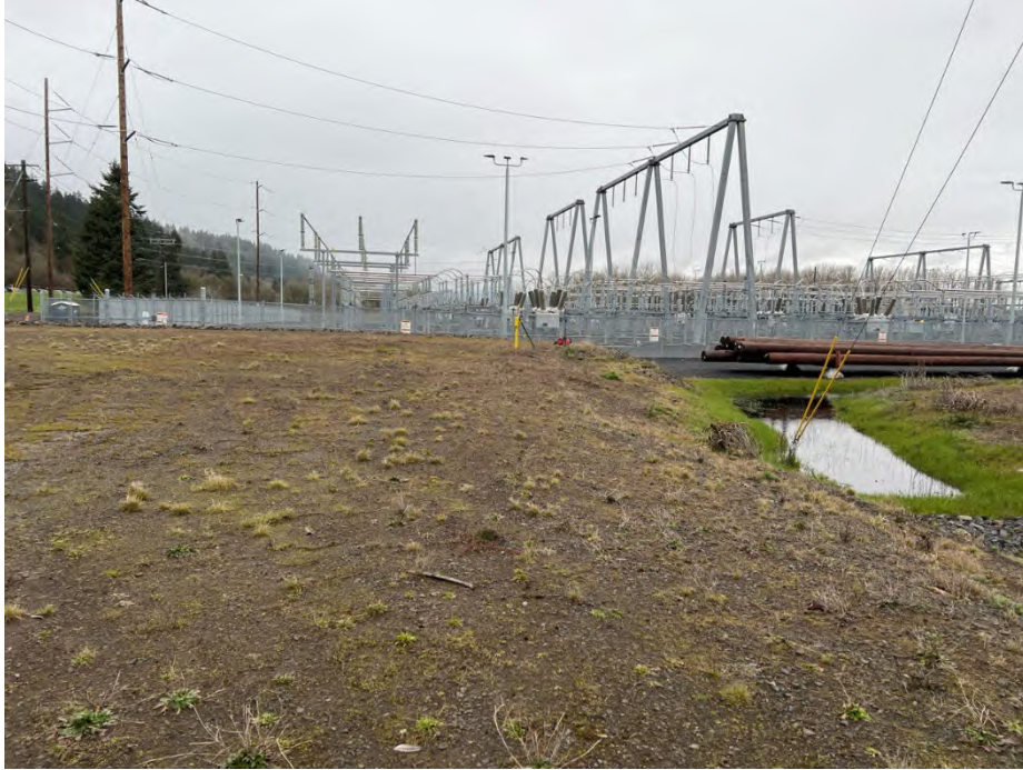
Photo 43 Stormwater collection canal (Ditch 1) located south of Harborton substation. Parallels substation fence line outside southern fence boundary. Date: 03/11//24 Direction: North
