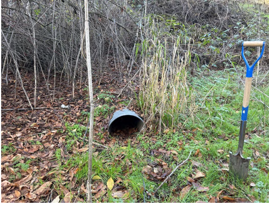
Photo 12b Culvert placed beneath adjacent road grade, no signs of recent flow. Date: 11/08/23 Direction: North
