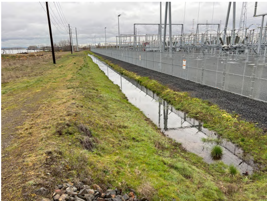
Photo 44 Stormwater collection canal (Ditch 2) located north of Harborton Substation. Date: 03/11//24 Direction: Northwest
