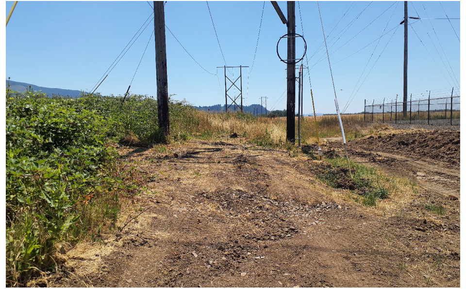
Photo 18. Category 6 Urban and Mixed Environs - transmission line and disturbed area adjacent to existing substation. 6/28/2023.
