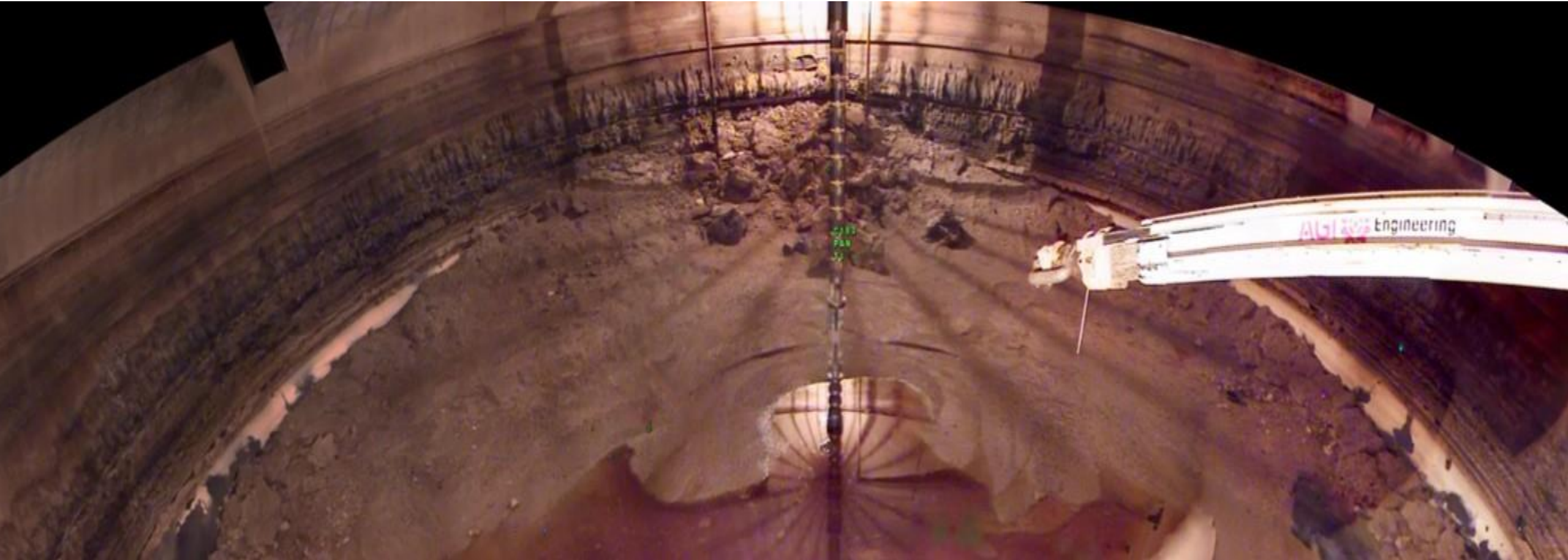
Tank C-102 – difficult sludge heel
