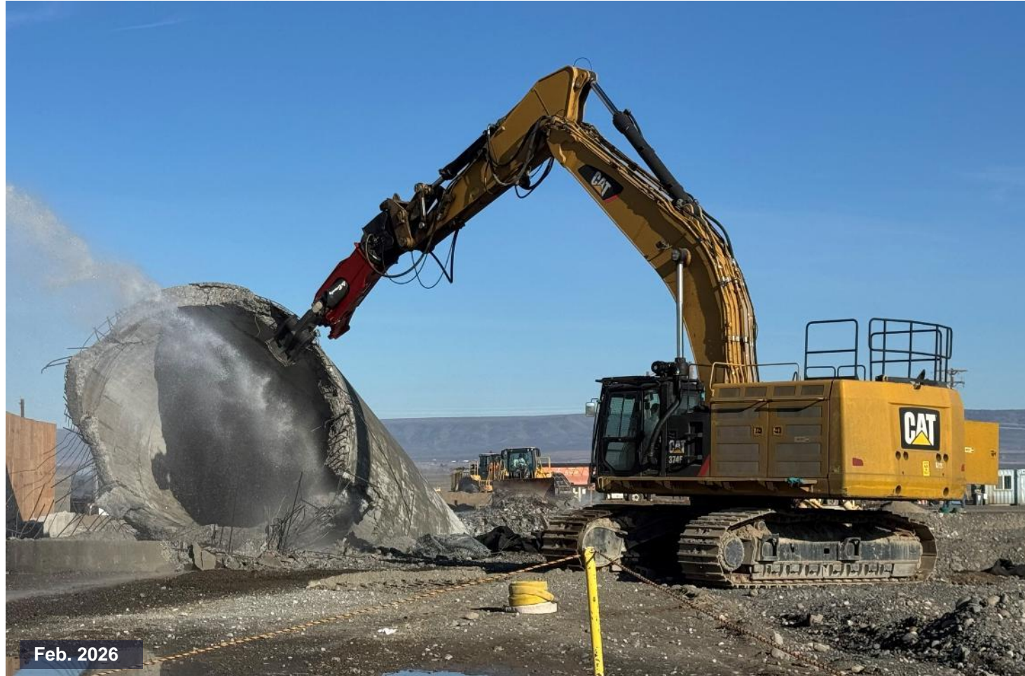
Reducing the size of the exhaust stack for transport to the Environmental Restoration Disposal Facility.
