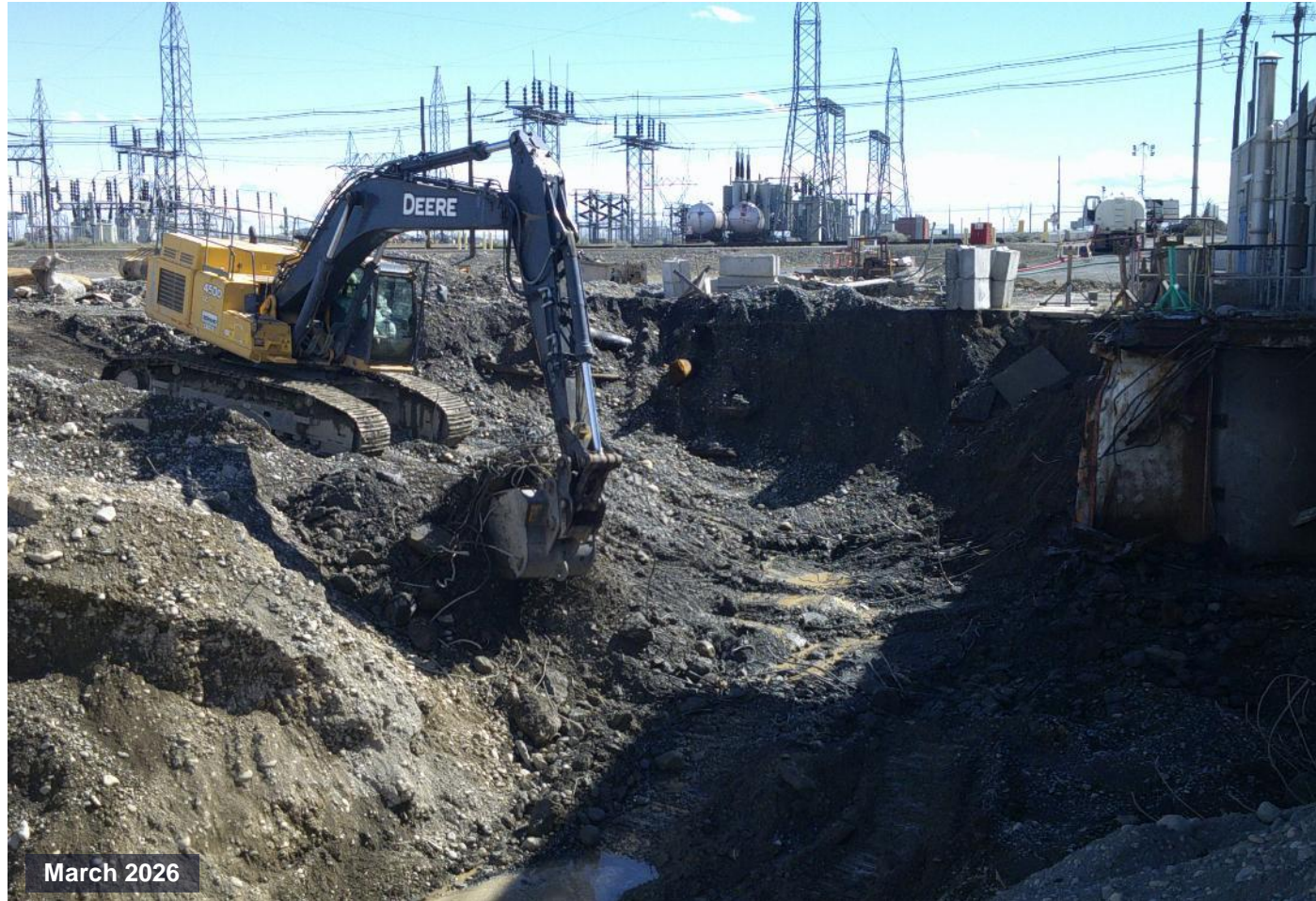
An operator works belowgrade to load out debris from the exhaust stack demolition.
