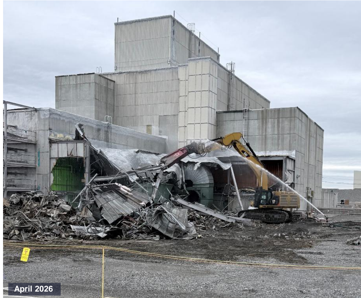
Demolishing the supply fan room on the southwest side of the reactor
