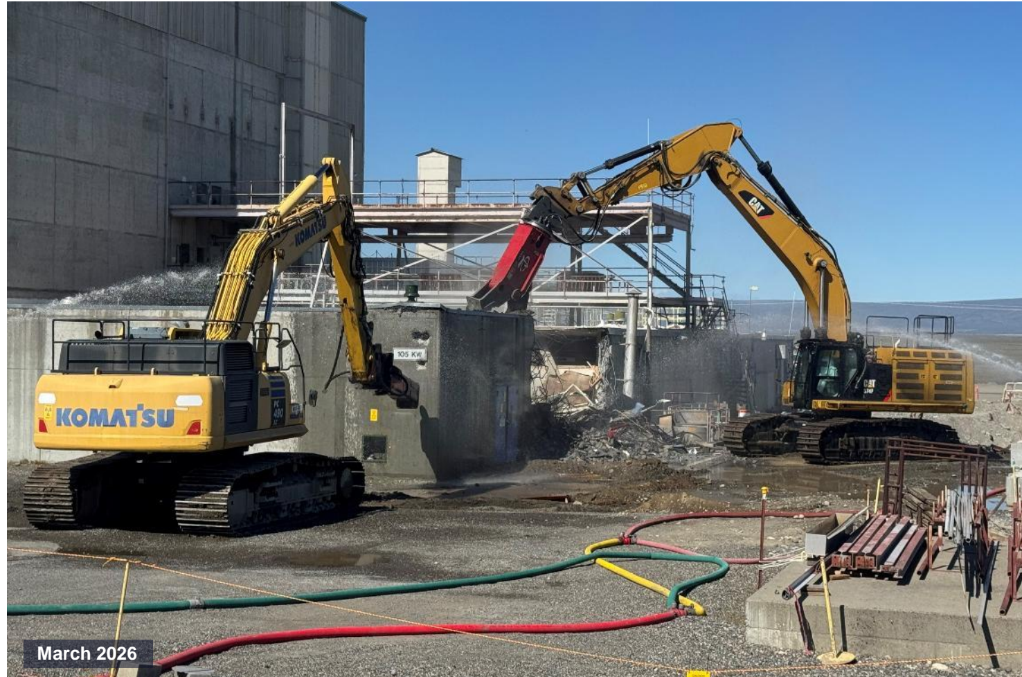
Demolishing the control room and administrative areas on the east side of the reactor.
