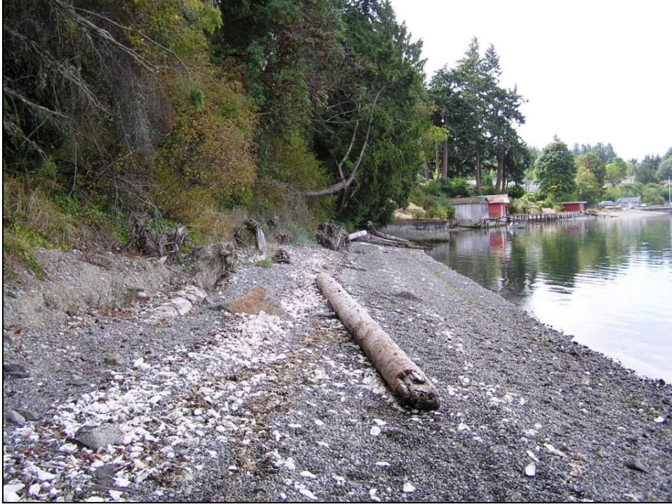
Figure 27: Kitsap Memorial Park, Southern Beach after bulkhead removal and soft shoreline stabilization.
