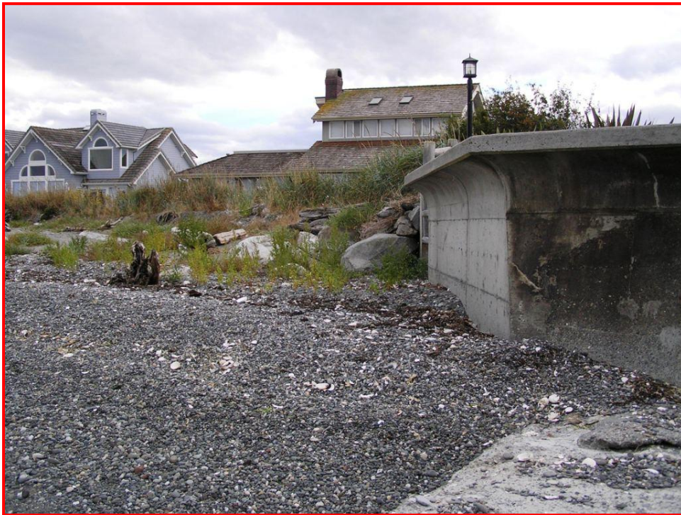
Figure 12: End erosion effects caused by this seawall resulted in the need for hard rock on the adjacent neighboring property. (Kelsey Gianou photo.)
