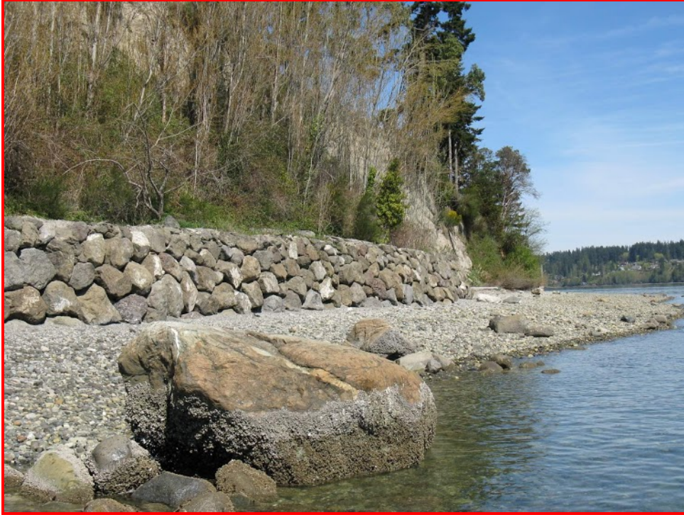
Figure 8: This rock seawall prevents erosion and the delivery of sediment to the beach. (Hugh Shipman photo.)
