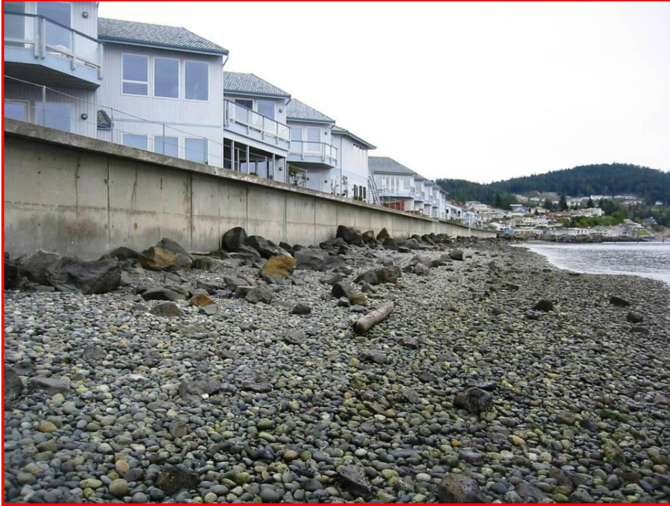
Figure 10: This seawall and riprap on a spit does not allow for natural accretion and erosion cycles of the beach. (Hugh Shipman photo.)
