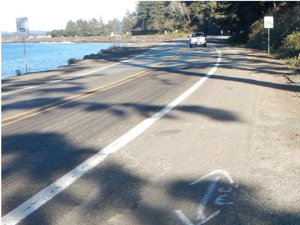
Widened paved/gravel shoulder used by OHV southeast side of road (looking Northeast)
