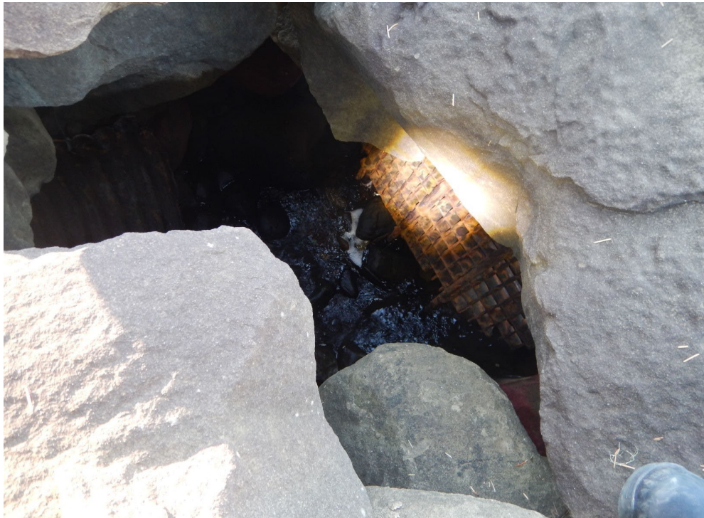
Unnamed stream south of Lighthouse Drive - culvert outlet into bays rocky shore
