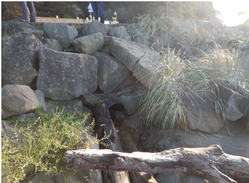
Unnamed stream outlet pipe at Winchester Bay Sanitary District (looking Southeast)
