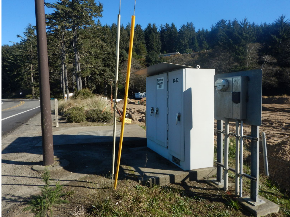
Sanitary pump station vaults and control panels (south side looking East)
