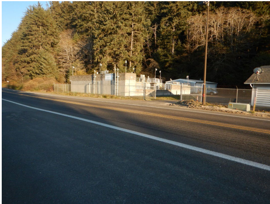
Sanitary wastewater treatment plant and maintenance facility (looking East)
