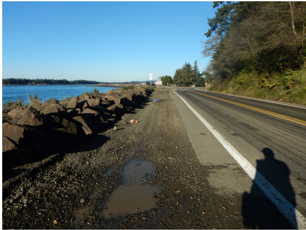
Widened gravel shoulder with rutting, ponding, and erosion (looking North)
