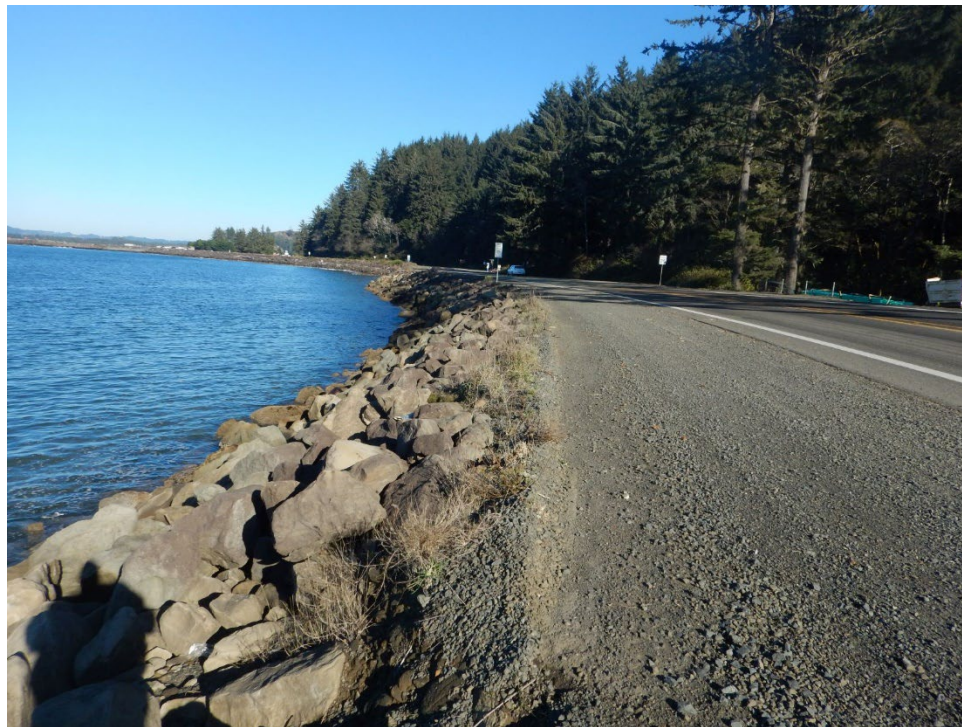
Widened gravel shoulder used by OHV directly along rocky shoreline (looking East)
